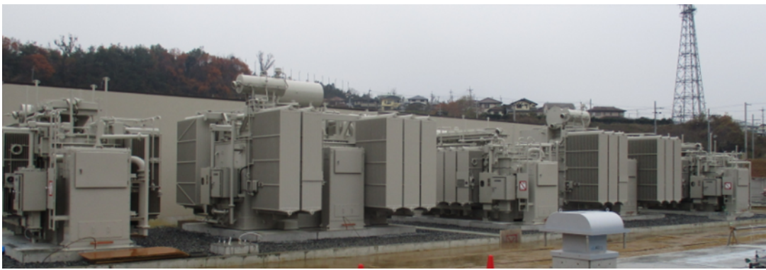
Fig.1 Substation applying transformers with rapeseed oil
