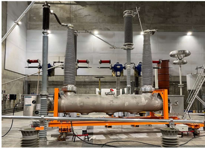
Figure 1: GIS 420kV Circuit-breaker C4FN at CERDA test Laboratory
