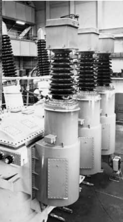
Figure 4.63(a) Three single-phase, fully insulated tapchangers fitted to the 132 kV tapping points of a 240 MVA, 400/132 kV autotransformer (Hawker Siddeley Power Transformers Ltd)
