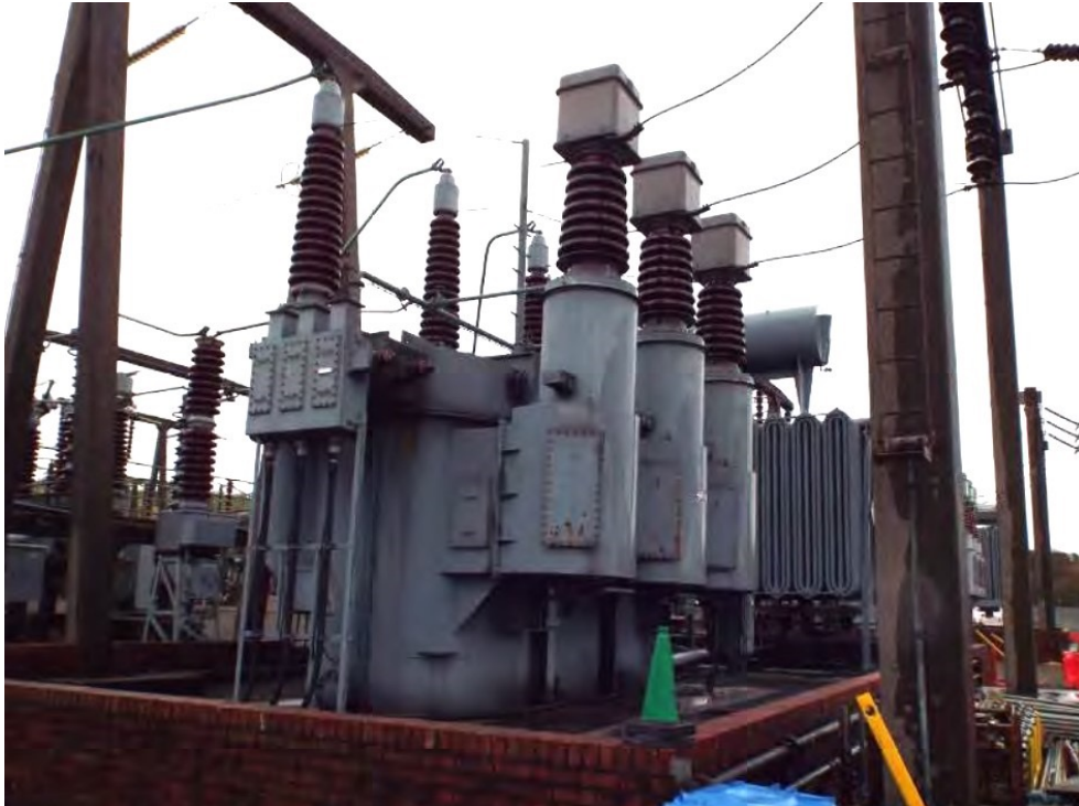
1967, line end tapchangers on top of bushings
