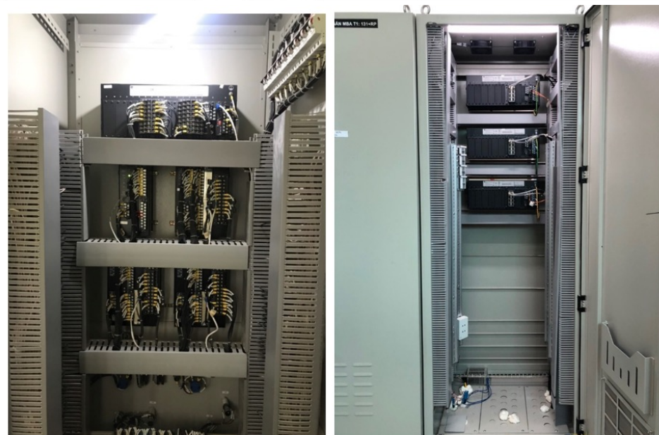
Figure 9: Protection panel at a typical conventional substation vs protection panel at 110KV Nghi Son Digital substation
