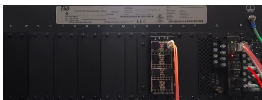
A typical P&C IED Device (Digital substation)
