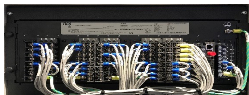
A typical P&C IED (Conventional substation)
