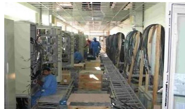
A typical conventional substation
