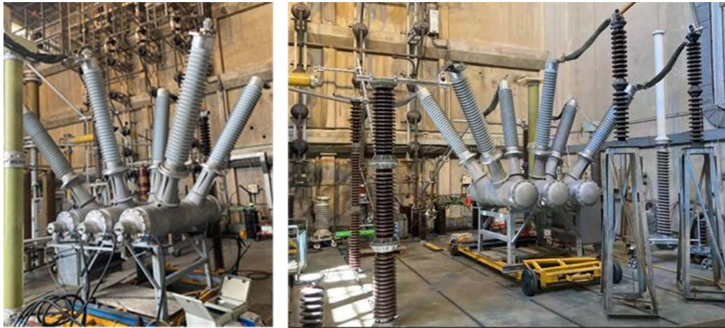
Figure 3. Dead tank 145g 3 during power breaking tests at CERDA.
