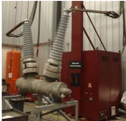
Figure 6: Dead tank 145g 3 during temperature rise test at 3000 and 4000 A.
