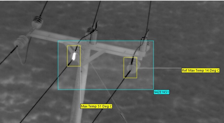
Thermal Image of a Pole
