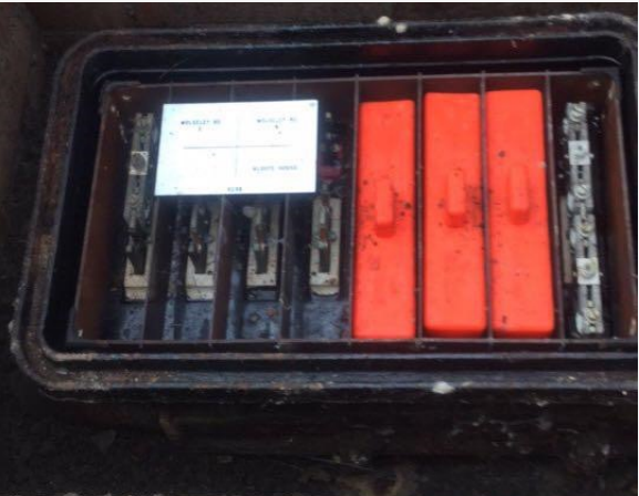
The Inside of a Link Box
