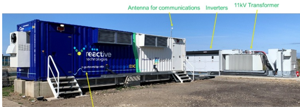
Container houses ultracapacitor cells and modules, control system, cooling system, fire detection and suppression
