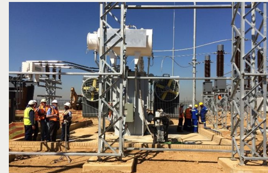
Substation field trip for training
