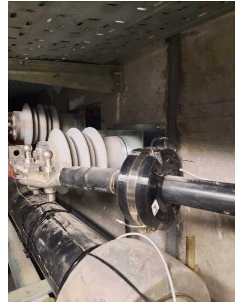
Sheath current monitoring CT at a cable joint
