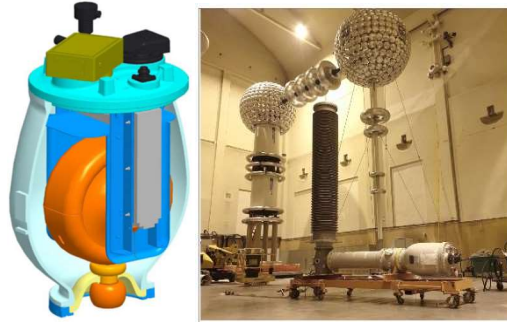
Figure 8 - SF 6 or dual-gas voltage transformer arrangement in test laboratory
