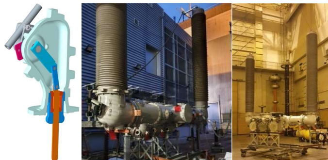
Figure 7 - SF 6 or dual-gas earthing switches arrangement during induced current test in laboratory
