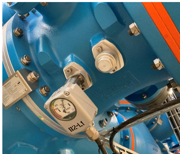
Figure 3 – Densimeter installed on GIS compartment
