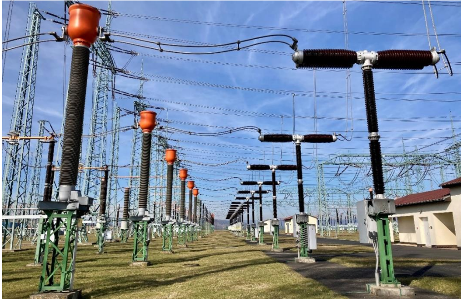
Fig. 7 Different types of current transformers and circuit breakers in 420 kV AIS substation filled with SF6
