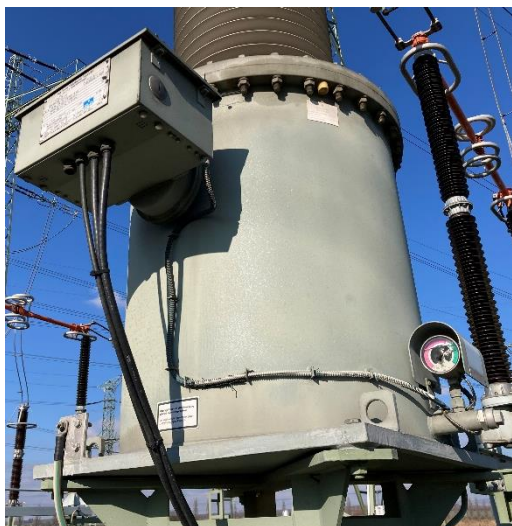
Figure 2 – Densimeter installed on VT in AIS
