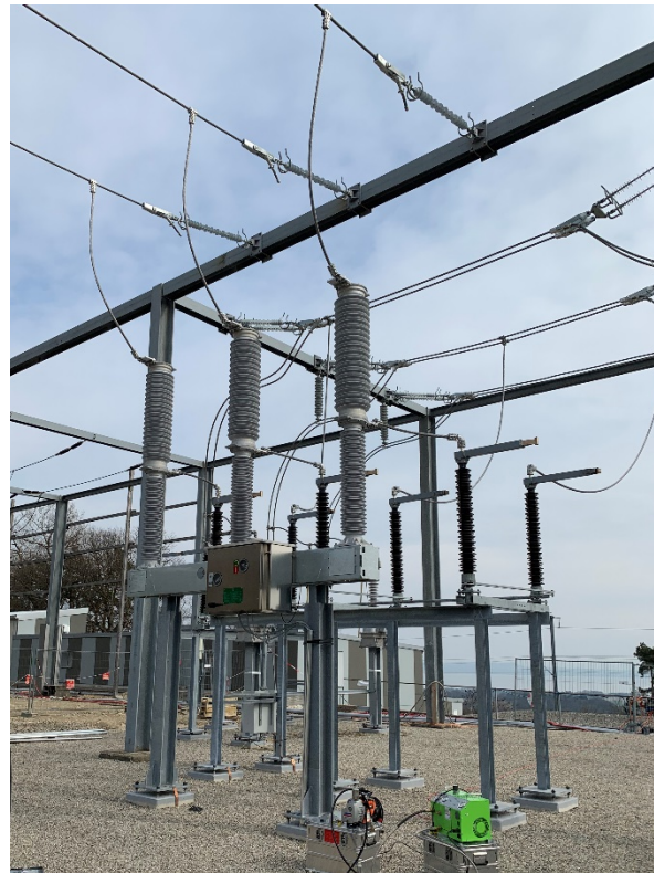
Figure 1 – 145kV 40kA C4-FN gas mixture circuit breaker installed on Planchamps Site in Switzerland
