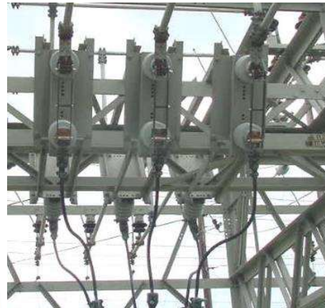
15 kV 600 A Recloser Disconnects three single pole switches
