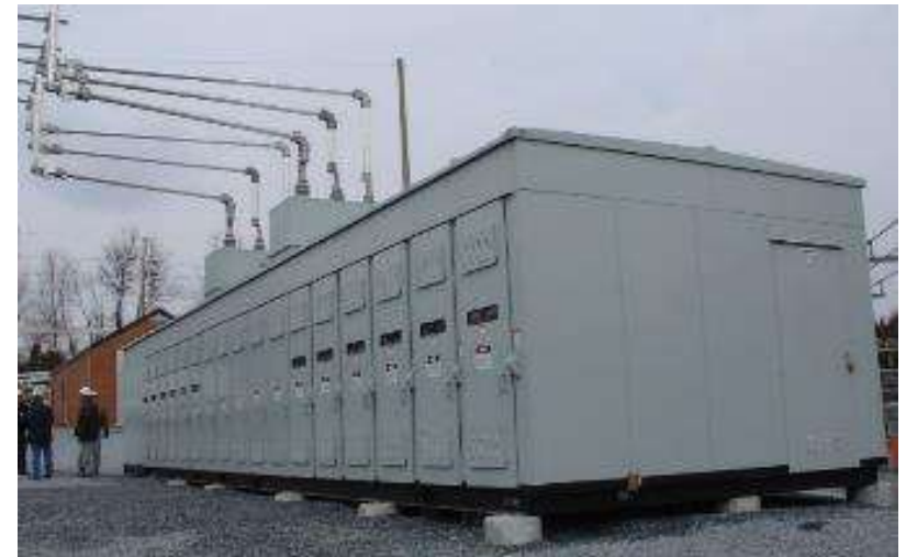
Example: 15 kV 3000 A bus outdoor walk-in sheltered aisle with 12 single high breaker cubicles in a single row and UG feeder exits
