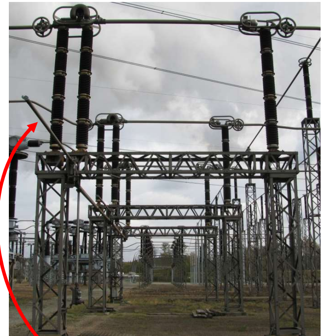
Earthing or Grounding Switch in the “open” position
