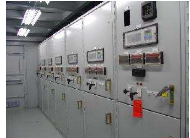
Example: 15 kV 3000 A bus outdoor walk-in sheltered aisle with 12 single high breaker cubicles in a single row and UG feeder exits
